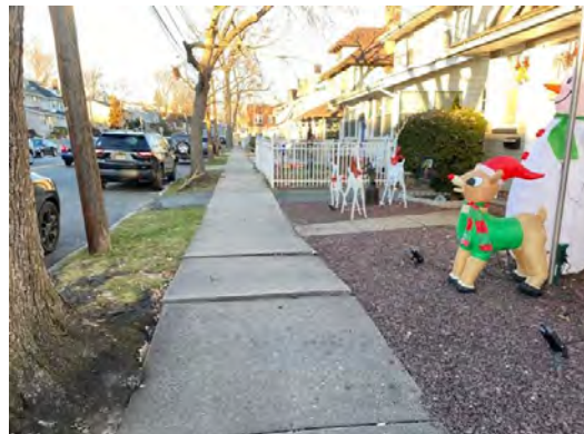
Raised sidewalk is trip hazard
