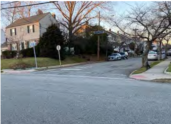
Faded crosswalk, misaligned dome pads
