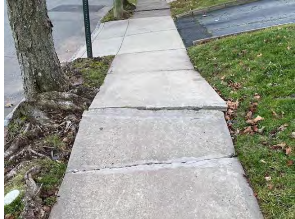
Uneven & cracked sidewalk
