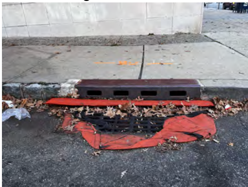
Drain needs repair & cleaning
