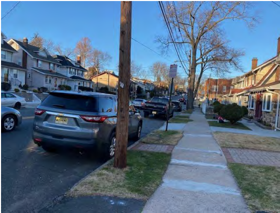
Uneven sidewalk is trip hazard
