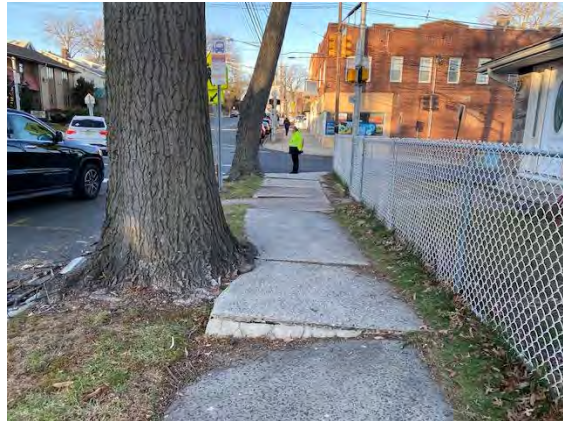
Raised sidewalk is a trip hazard
