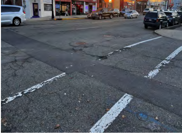
Crosswalk & road repair needed
