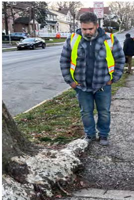
Raised sidewalk is trip hazard
