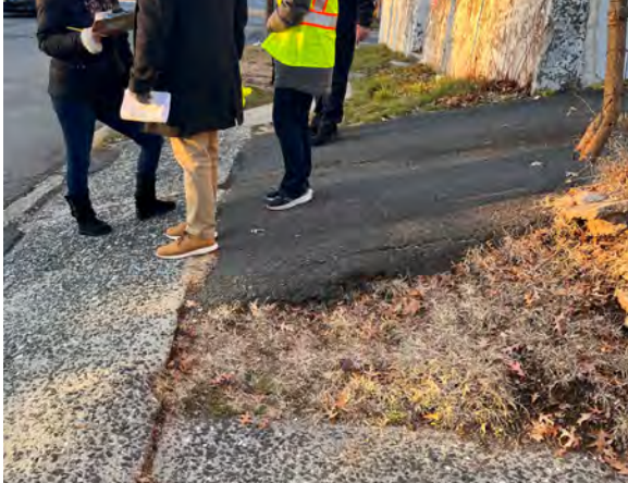
Sidewalk slanted towards road
