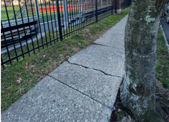
Cracks in sidewalk from tree uprooting
