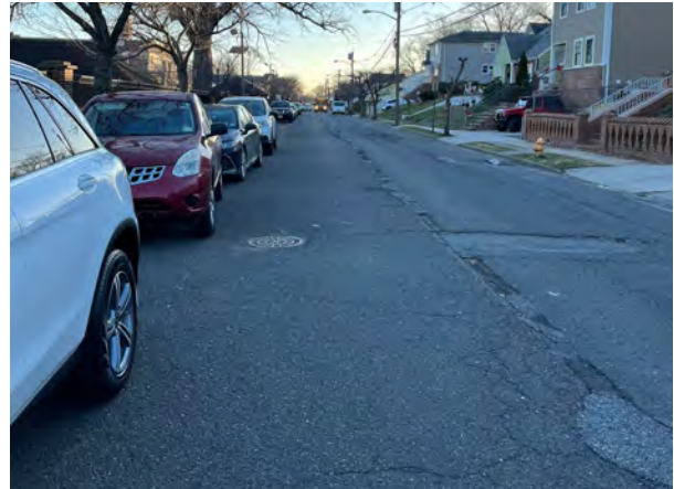
Cracks & potholes looking south
