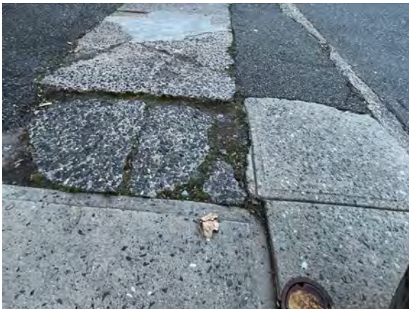
Cracked & Uneven Sidewalk
