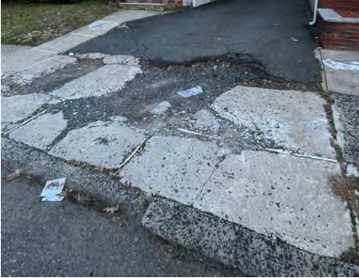
Pothole & cracks in the sidewalk
