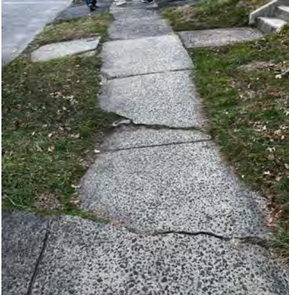
Sidewalk in need of repairs
