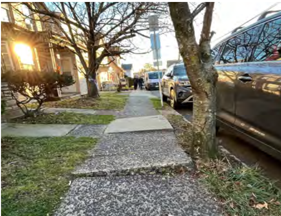
Uneven sidewalk & low hanging branches
