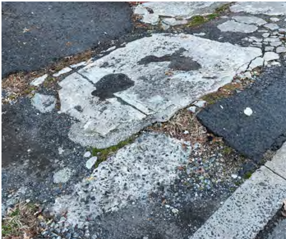
Cracked & uneven sidewalk
