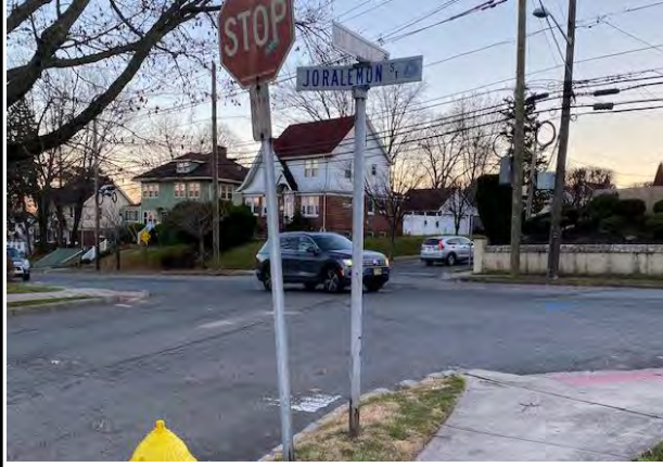
Faded crosswalk & stop bar paint
