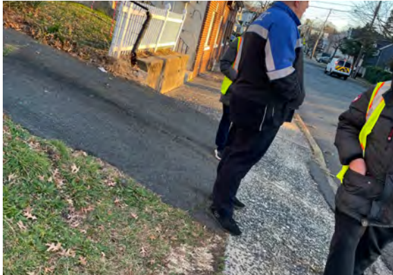
Sidewalk slanted/sloped towards road
