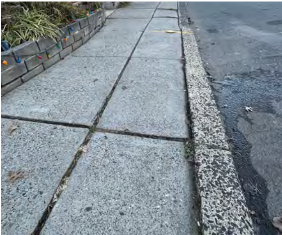
Wide gaps in sidewalk
