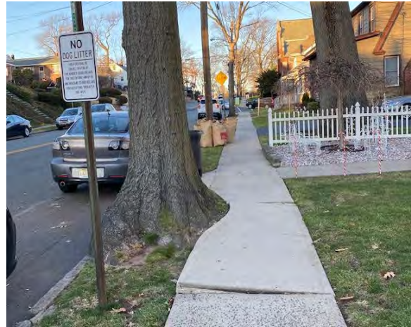
Raised sidewalk is trip hazard
