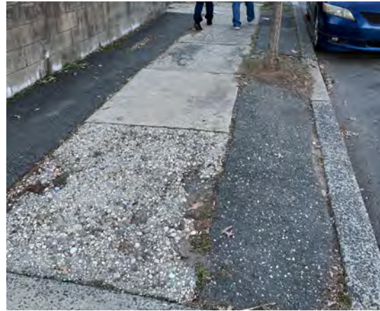
Sidewalk in need of repairs
