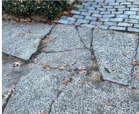
Cracks in sidewalk
