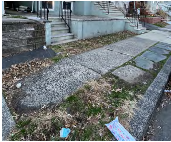
Cracked & uneven sidewalk
