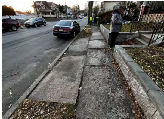
Sidewalk in need of repairs
