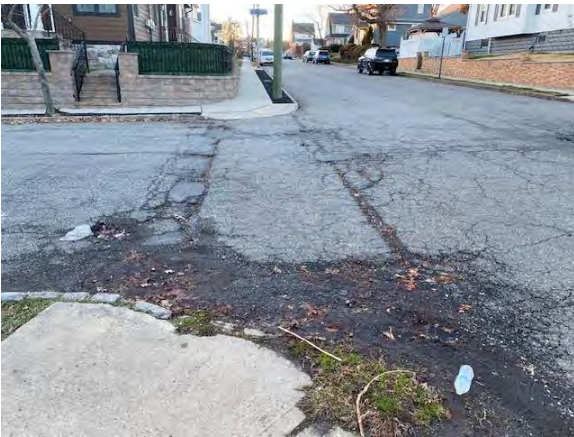
Grass & debris near sidewalk ramp
