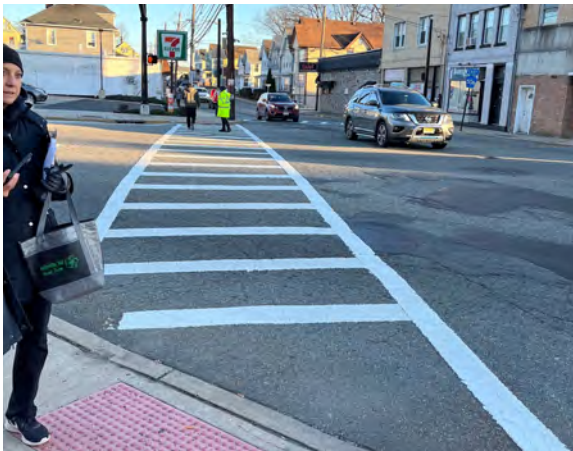
Dome pad is misaligned
