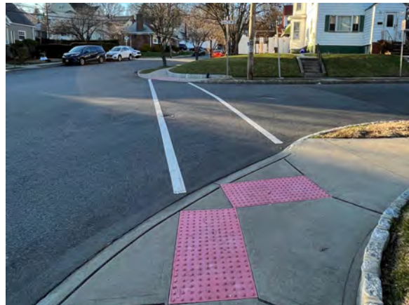
No stripes in crosswalk
