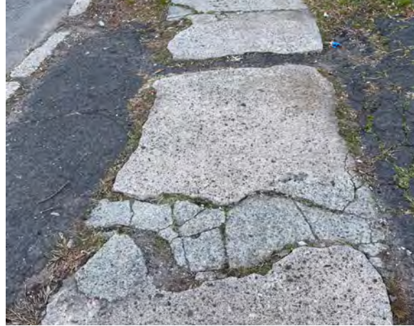
Badly damaged & cracked sidewalk
