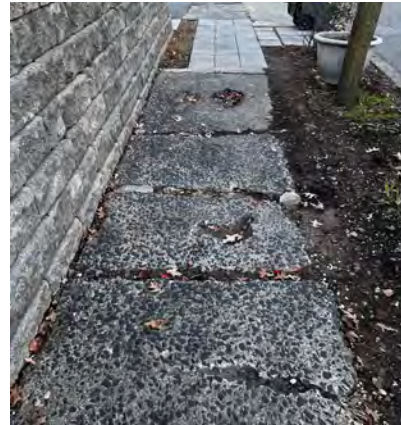
Sidewalk in need of repairs
