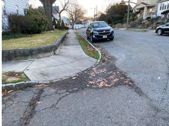
Debris & water gathering near sidewalk
