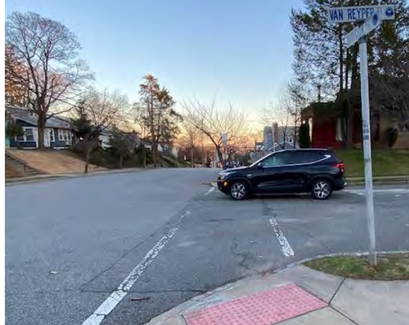
Faded crosswalk, misaligned dome pad
