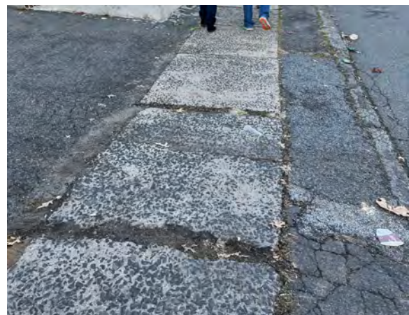
Cracked & uneven sidewalk
