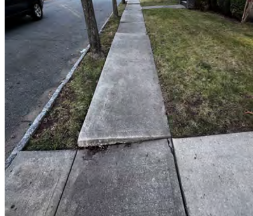
Raised sidewalk is trip hazard
