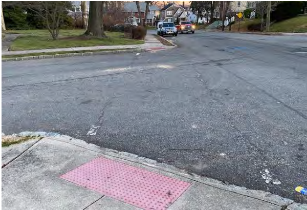
Misaligned dome pad
