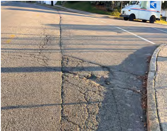
Cracks in the road where cyclists ride
