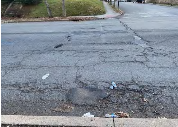
Faded crosswalk, many cracks in road
