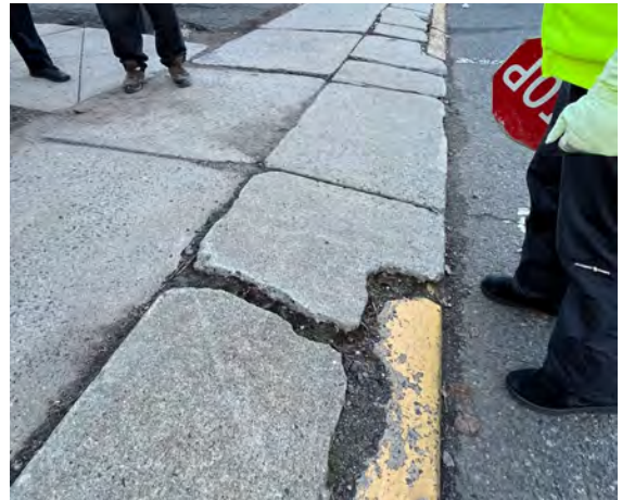
Cracked sidewalk with wide gaps front of school
