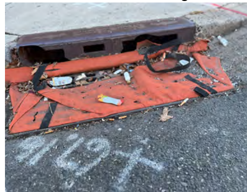
Drain needs repair
