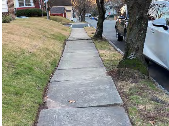
Sidewalk is uneven
