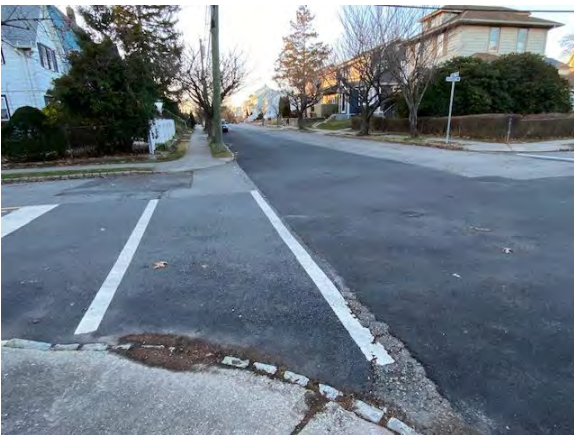
Crosswalk unfinished, no dome-pads
