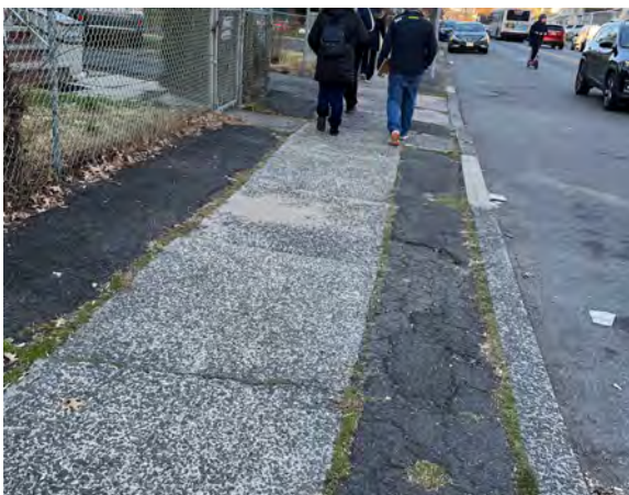
Cracked asphalt on the sides
