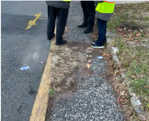
Sidewalk in need of repairs
