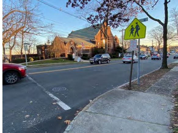
Sidewalk uneven from tree roots
