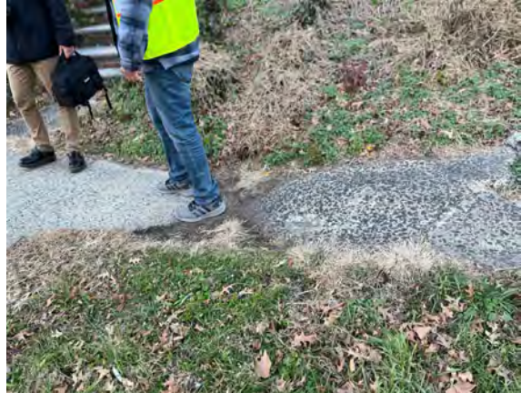
Sidewalk in need of repairs
