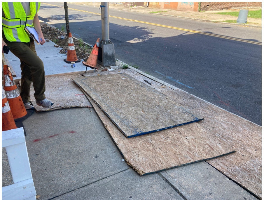
Figure 31 - Unsafe conditions during sidewalk construction
