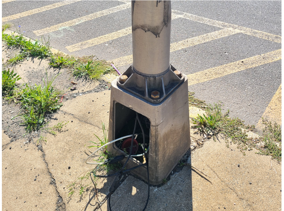
Figure 30 - Light pole with exposed wiring
