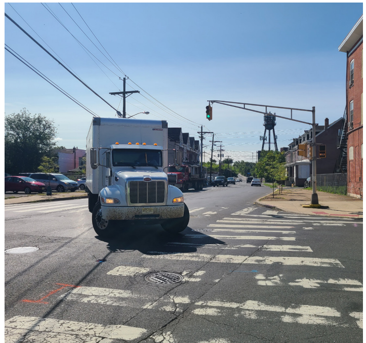
Figure 17 - Worn Crosswalks at N. Clinton Ave & N. Olden Ave
