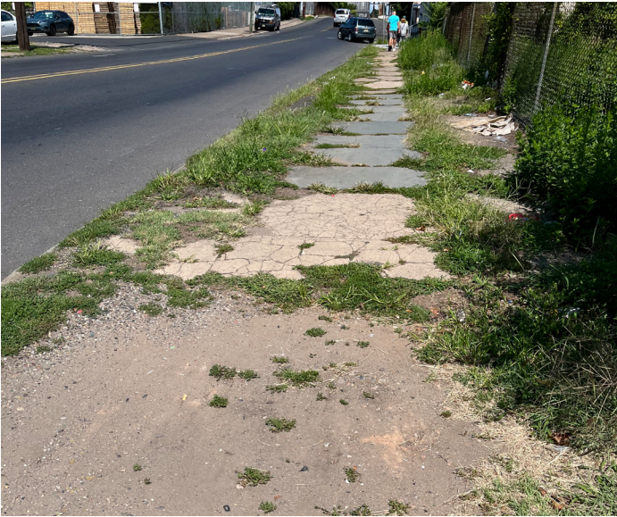
Figure 10 - Poor sidewalk condition on N. Olden Ave near Ward Ave.
