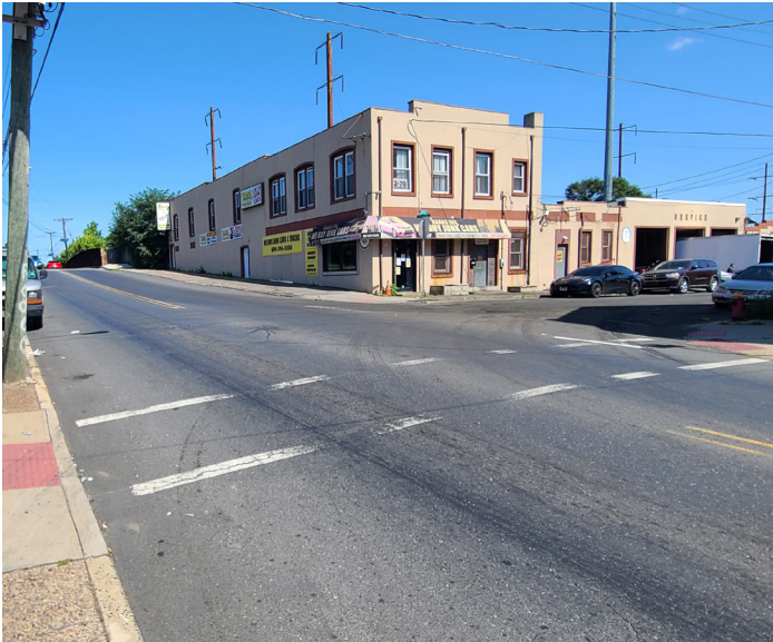
Figure 19 - Worn transverse line crosswalk across N. Olden Ave
