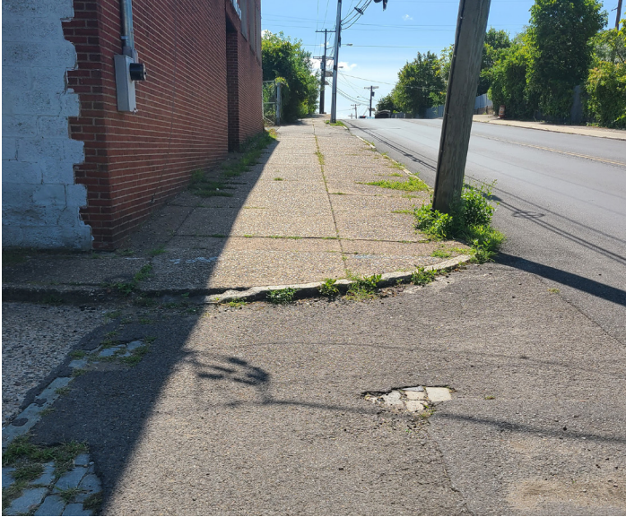
Figure 14 - Example of many curbs missing an ADA ramp
