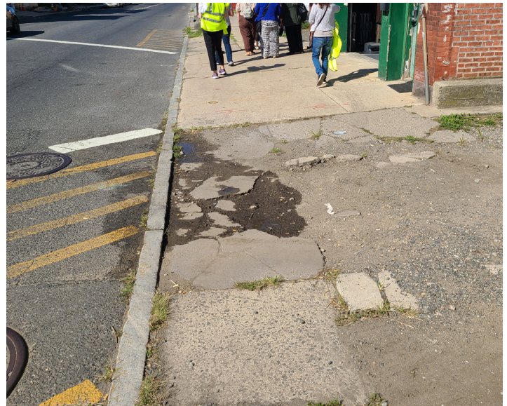
Figure 7 - Deteriorated sidewalks on N. Clinton Ave
