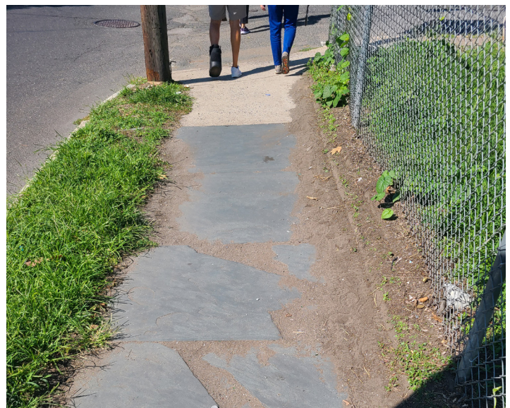
Figure 9 - Slate sidewalk at N. Clinton Ave & Eastburn Ave
