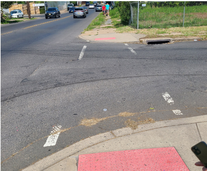
Figure 21 - Worn crosswalk at Ward Ave & N. Olden Ave
