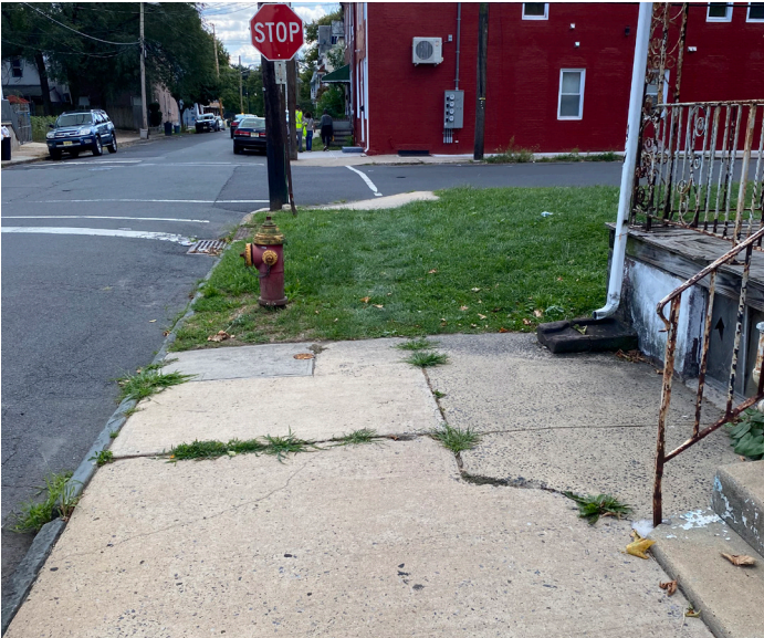
Figure 11 - Missing sidewalk at St. Joes Ave & Girard Ave
