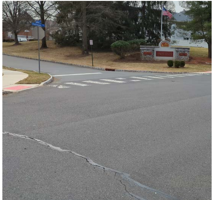
Figure 15 - Missing Crosswalk over Stephenson Rd at Gifford St
