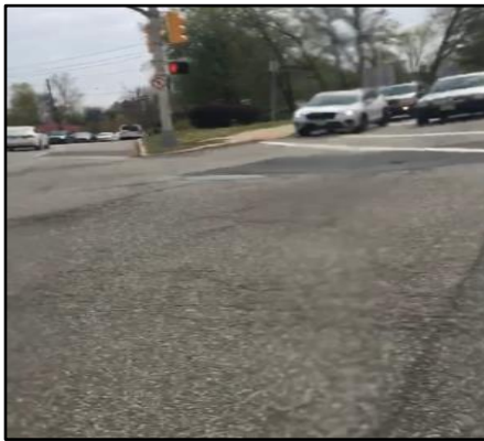
Long crossing distance and no stripes in crosswalk
