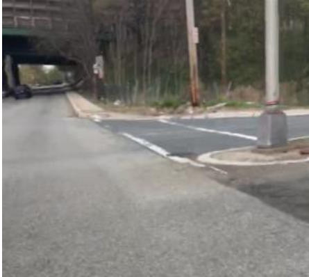
No stripes in crosswalk
