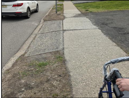
Sidewalk partly covered in dirt/debris
