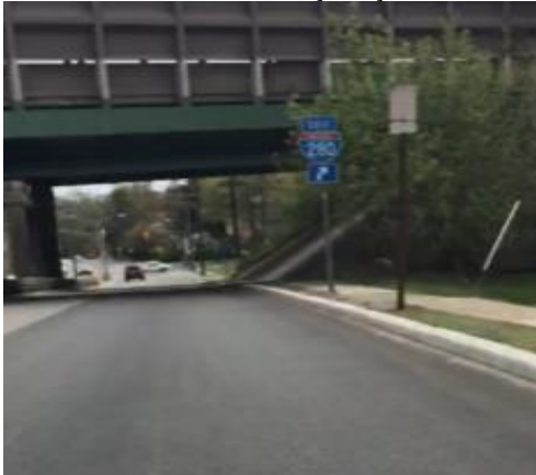
Sidewalk and road continue under RT 280 - add lighting
