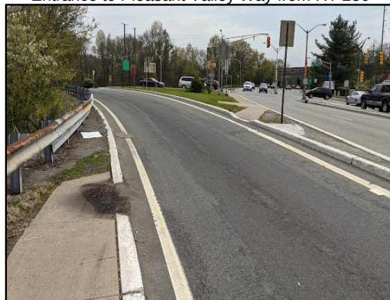
No crosswalk, water/debris accumulating at ramp
